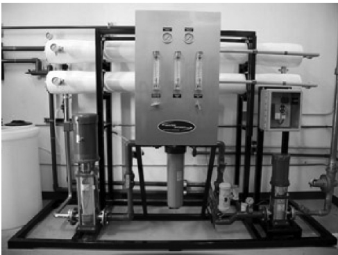
Reverse Osmosis Multi-stage pump supplies the pressure needed to push water through the membrane(s).
